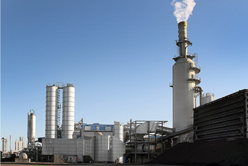
Comparable flue gas scrubbing plant with DeNOx stage and DeSOx scrubber constructed using concrete.
